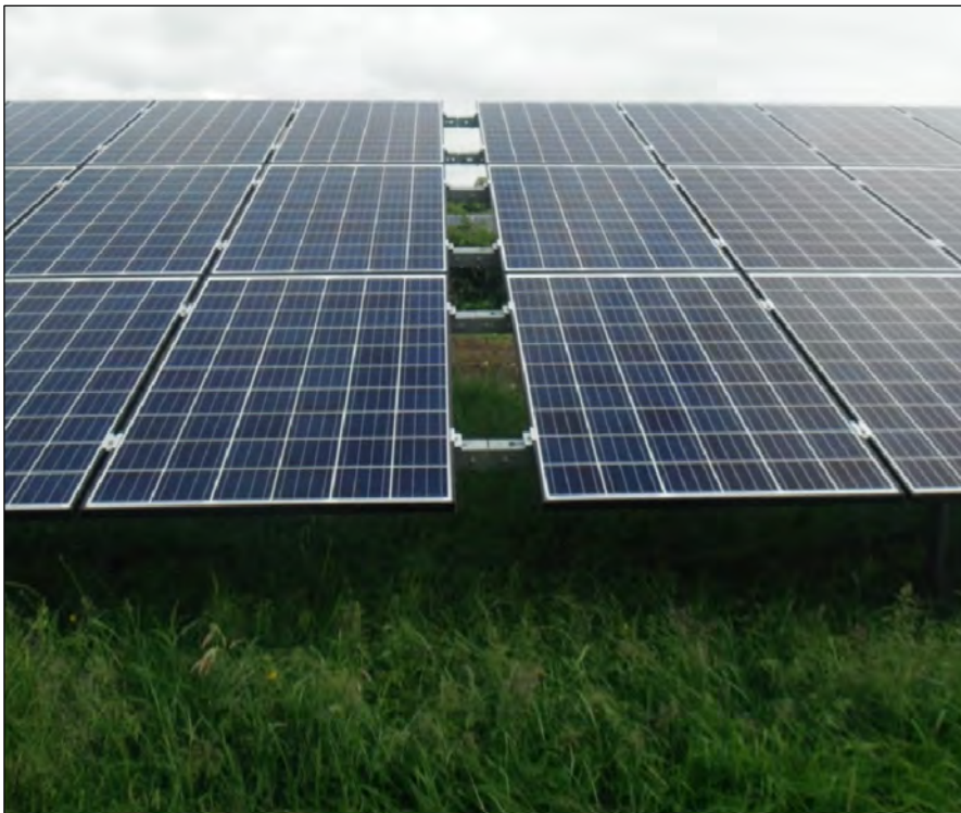
Figure 5.1 Photo of solar panels (front elevation)
