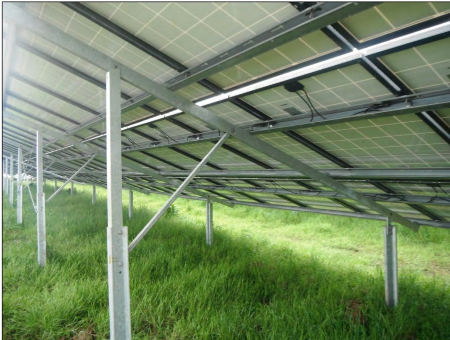
Figure 5.2 Photo of solar panels (underneath)
